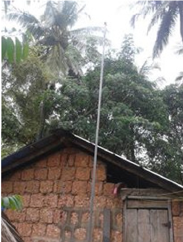
15ft pipe for gas emissions from septic tank
